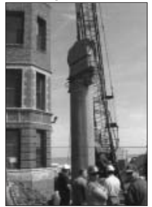
Workmen install caissons as foundation of the 25-unit indoor parking garage at 1200 W. Sherwin. The project is being completed by the developer, Nate Jarvinen, for owners of the condo units, to help relieve the parking congestion in the area.
